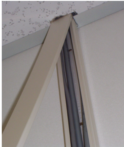
Fig. 4: The cables of two neighbouring coil rings (part of x- and y-coil) are placed in the same housing. The third cable is the connection cable between the z-coils which are in the ceiling and floor of the room.
